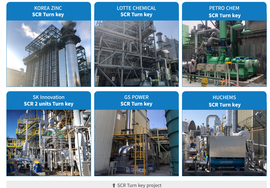
↑ SCR Turn key project
