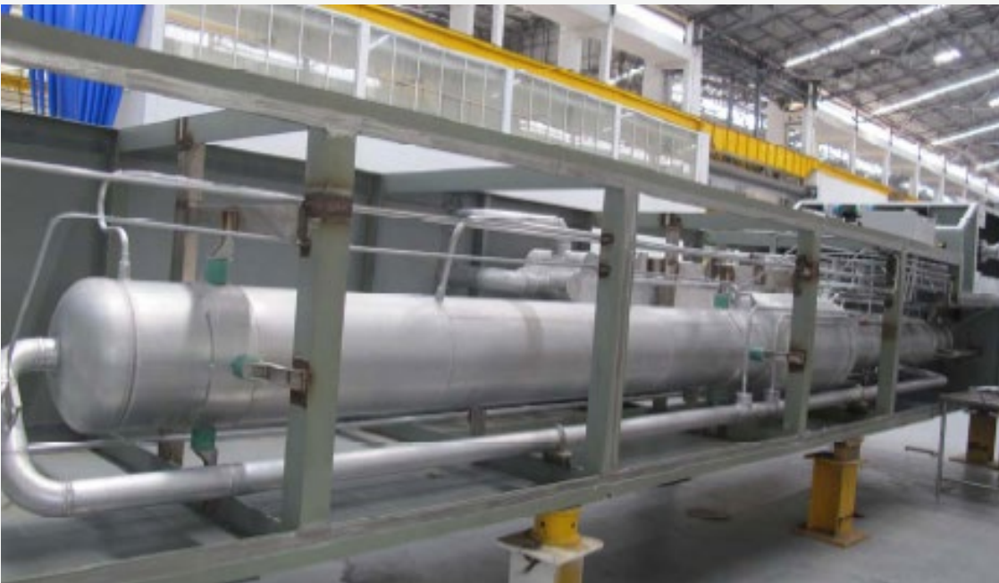
Cold box module internals
