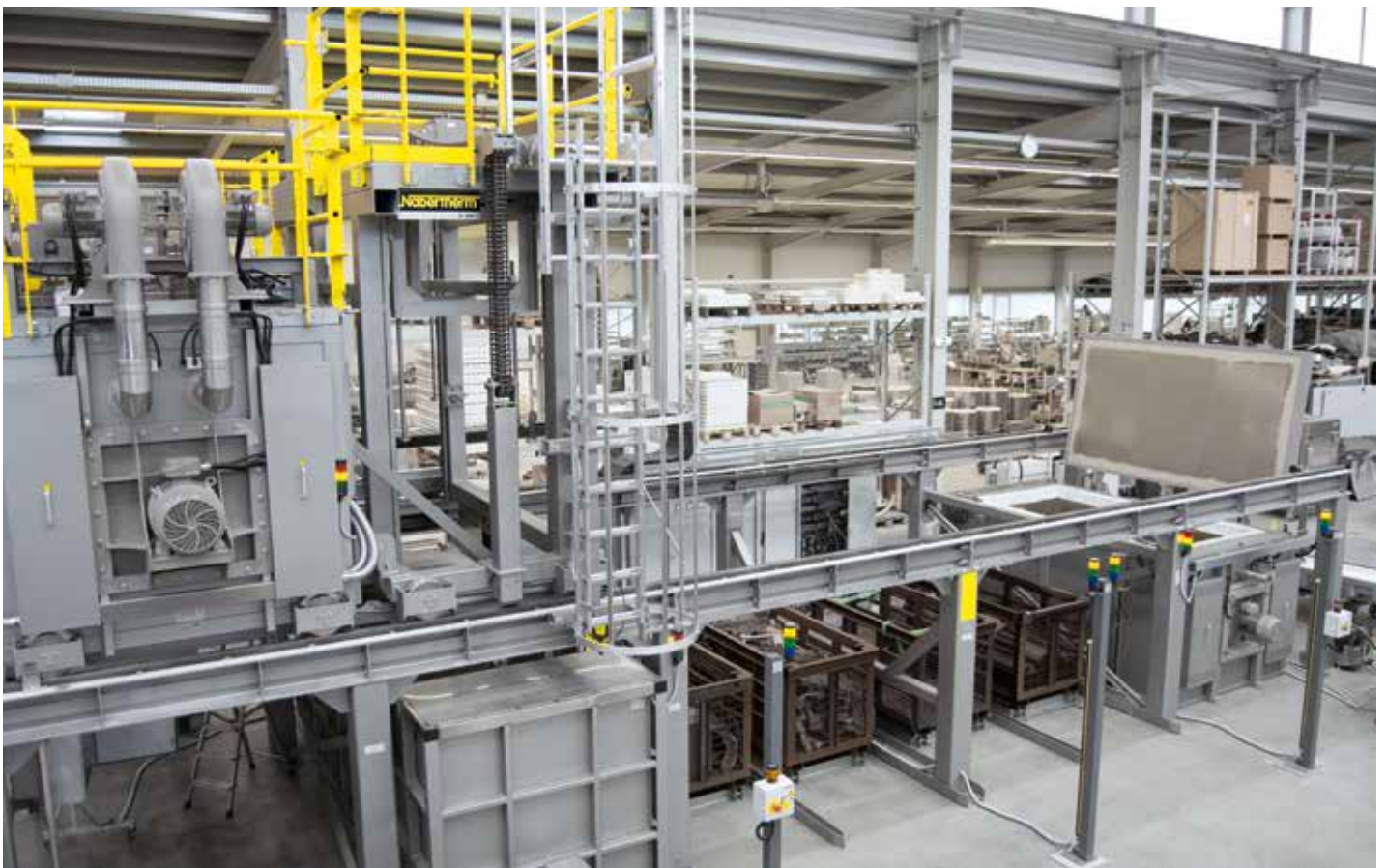
Movable drop-bottom furnace for solution annealing with pit-type furnace for artificial aging with four holding positions
