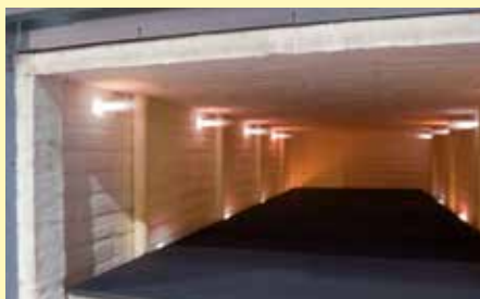
Furnace chamber with eight high-speed burners
