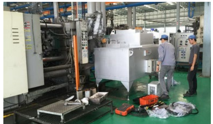
Installation & Tune up System
