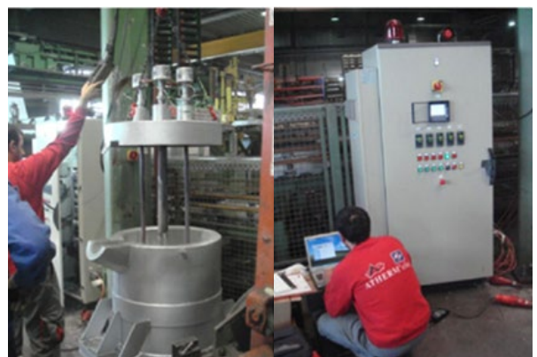
Technical assistance & Project management: Installation design phase assistance, commissioning and training assistance
