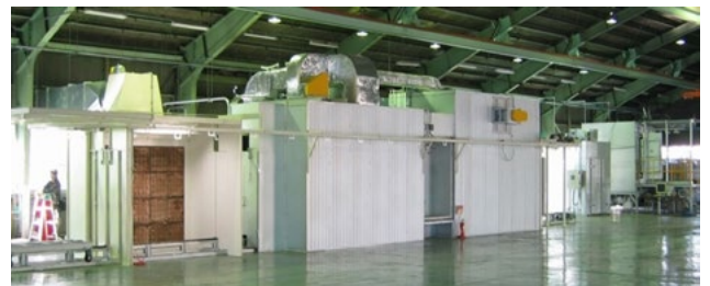
Continuous painting and drying furnace
