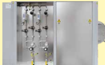
Gas supply system with mass flow controller
