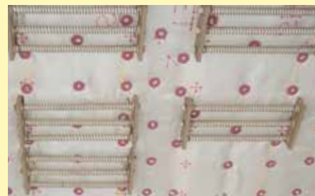
Fiber insulation covered with fabric to reduce dust in the furnace
