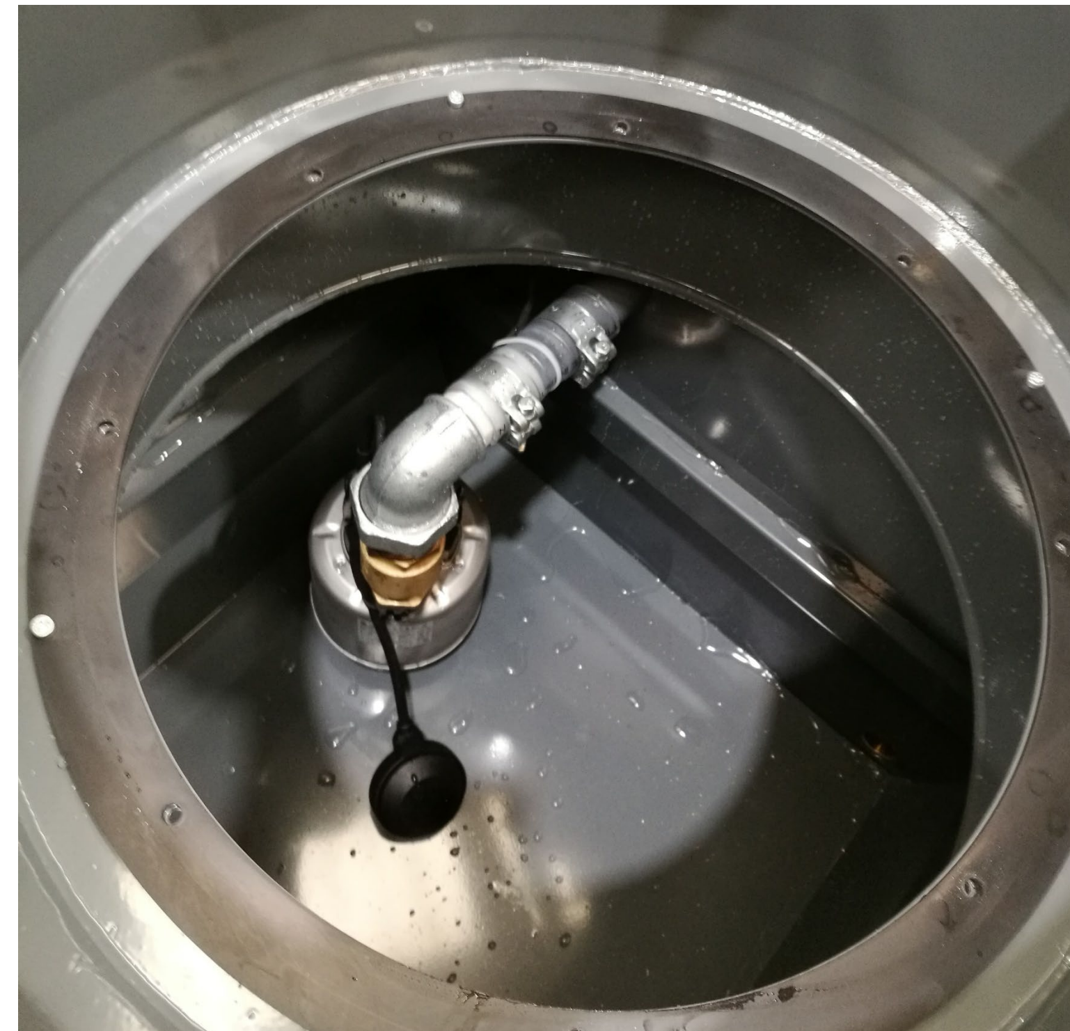
Automatic discharge maximum level is detected by a level sensor
