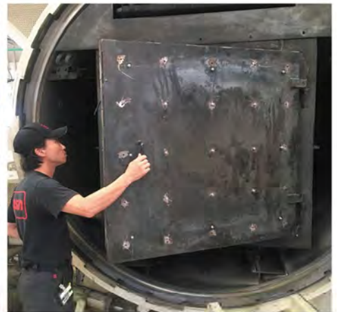
Install to furnace in customer factory
