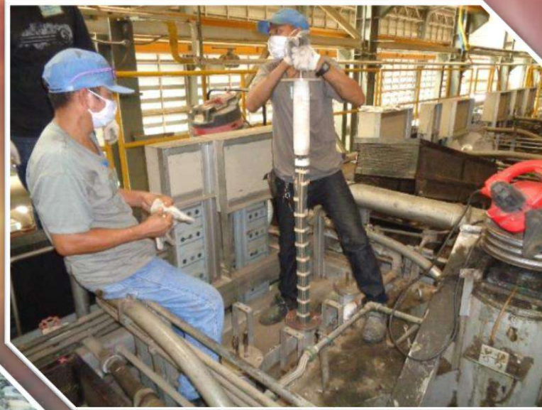
Checking of Radiant Heater
