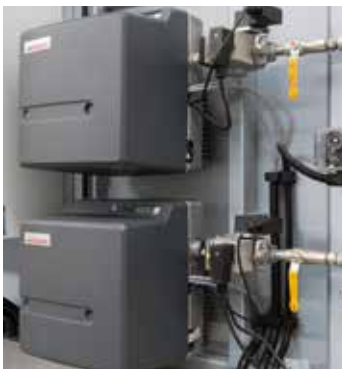
Gas burners for furnace heating and thermal afterburner
