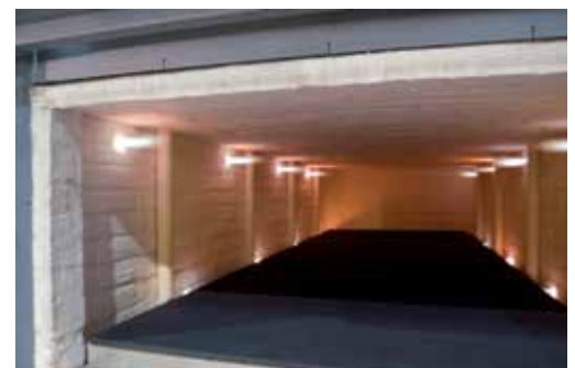
Furnace chamber with eight high-speed burners
