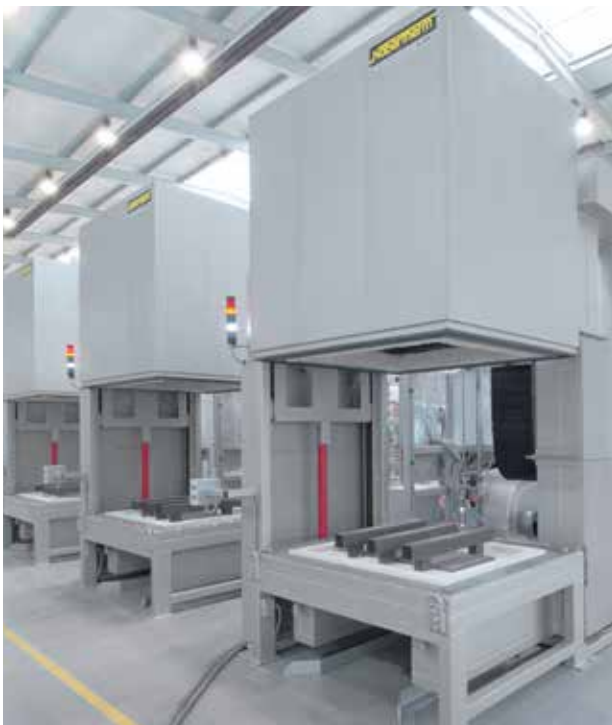
Production plant, consisting of 3 top hat furnaces HAS 1560/95S with sealed housing for operation with nitrogen. Including air/gas heat exchanger for reduced cooling times
