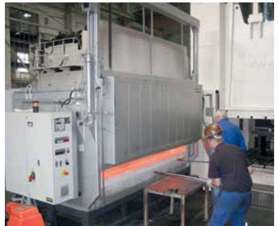
Chamber furnace N 1491/S in production
