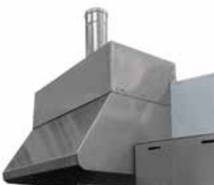
Exhaust hood above charging opening
