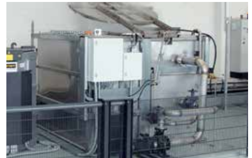
Quench tank with water integrated in a tempering plant for aluminium
