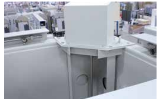
Protective gas supply as fire protection
