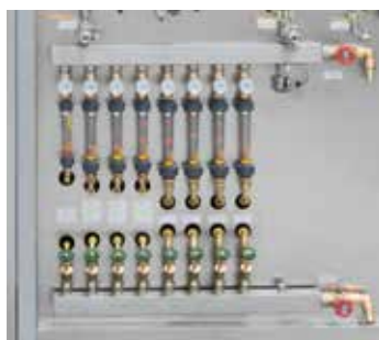
Cooling water distribution
