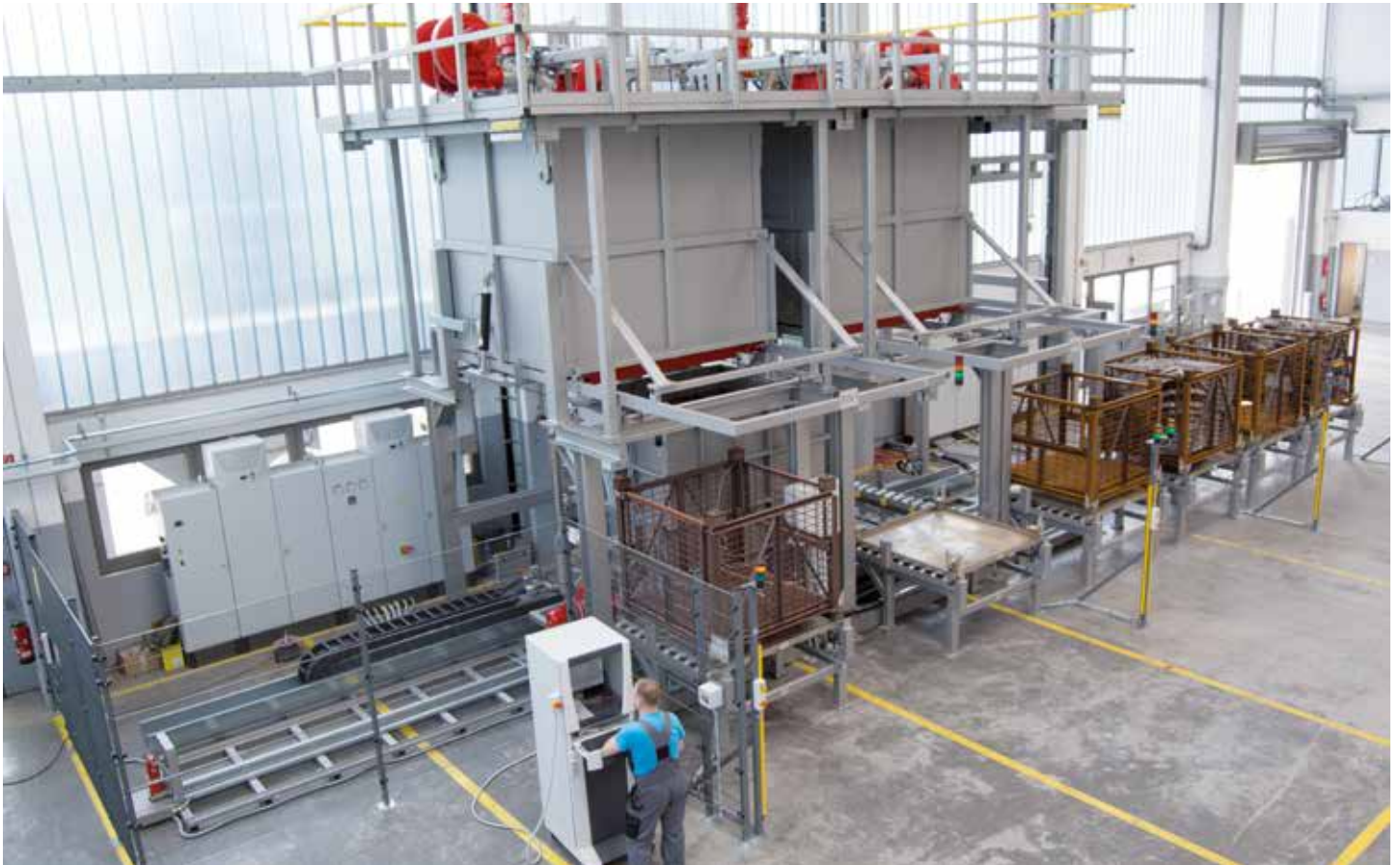
Fully automatic drop-bottom furnace plant, consisting of two drop-bottom furnaces, movable water bath and several loading and unloading positions
