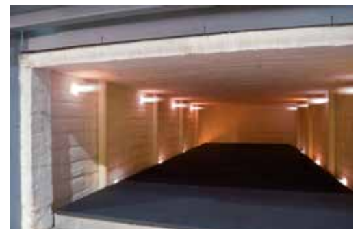
Furnace chamber with eight high-speed burners
