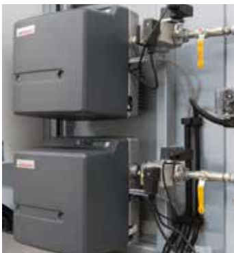
Gas burners for furnace heating and thermal post combustion
