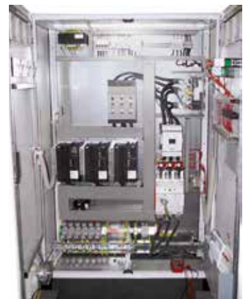
Switchgear with thyristors in phase angle operation for economic power consumption
