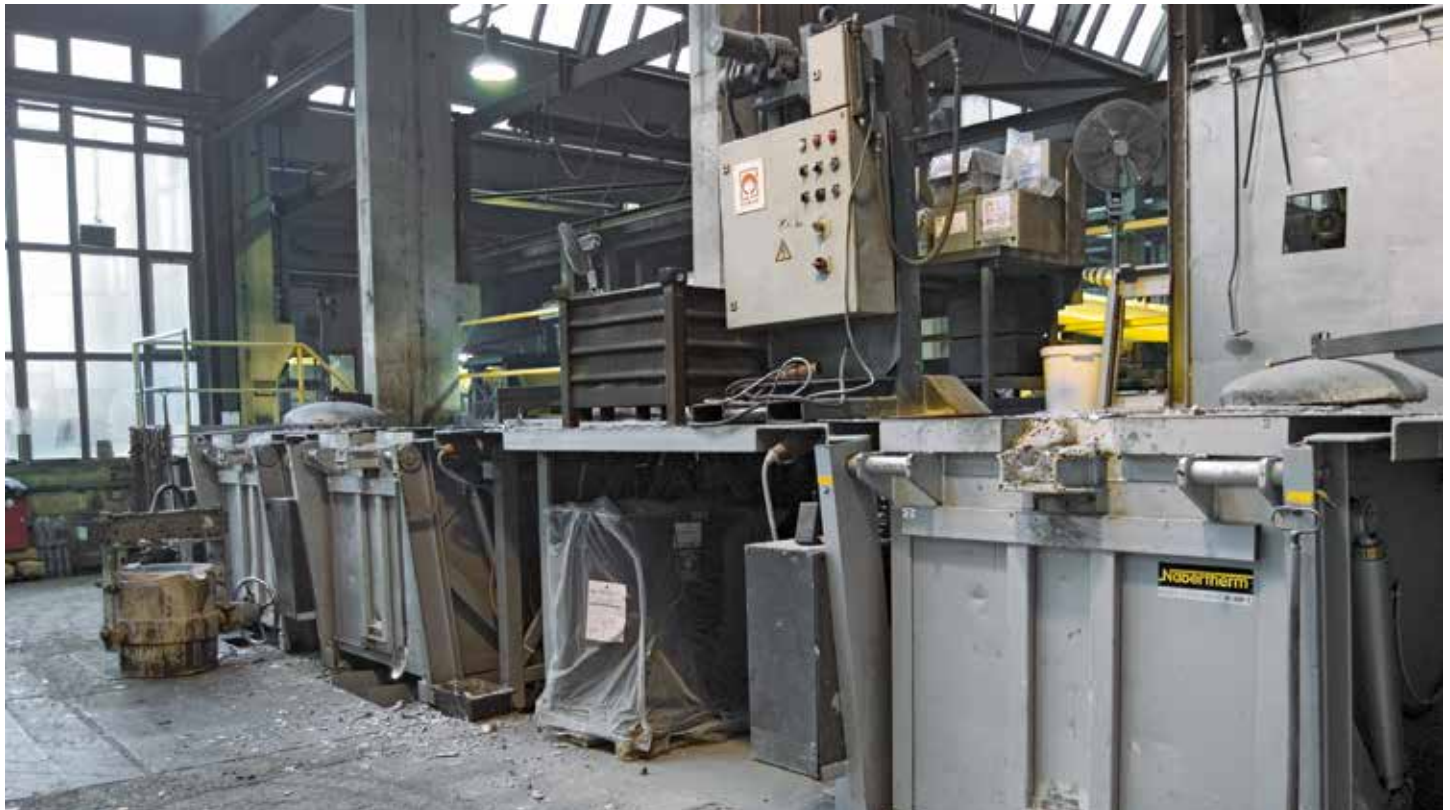
3 tilting furnaces K 300/12 with work platform for melting of aluminum
