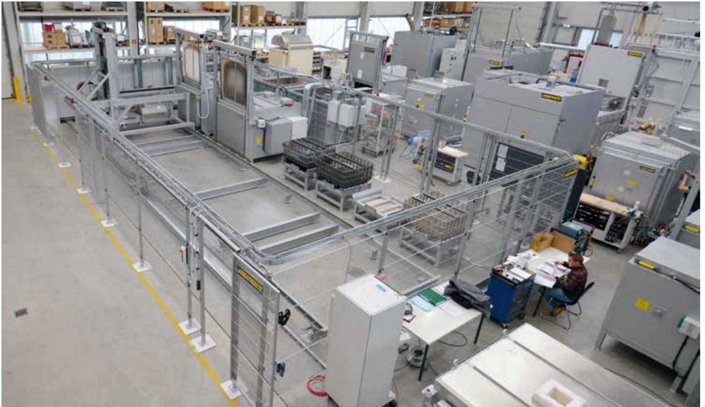
Fully automated tempering plant with two chamber furnaces, quench bath, conveyor system, and parking spots for four charge baskets
