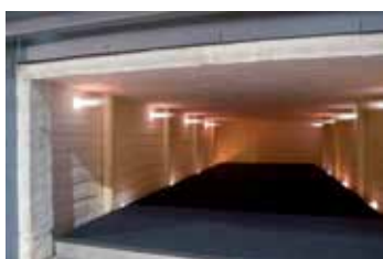
Furnace chamber with eight high-speed burners
