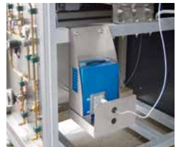
Acid pump for nitric acid
