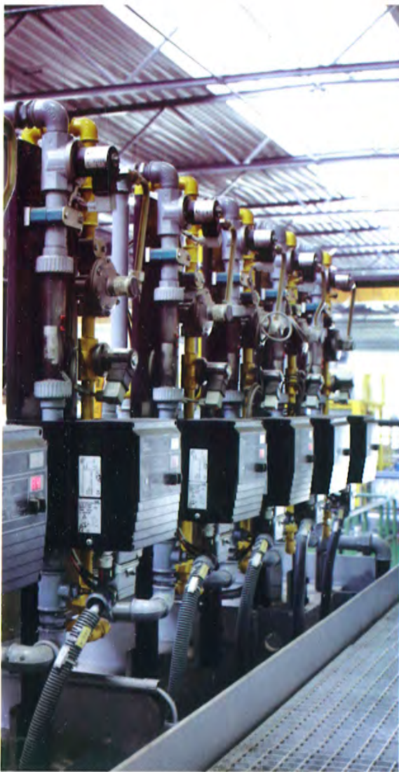
Mixing battery and control electronics of a Recon®-heating system
