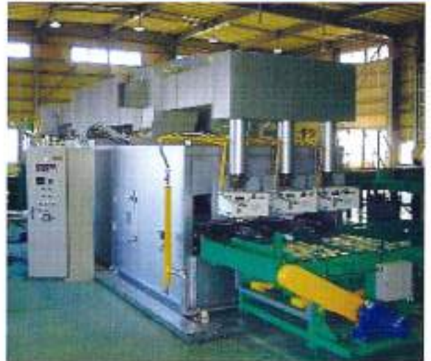
Continuous paint drying furnace for plastic parts Far-infrared burner BT-33NH x 6 units
