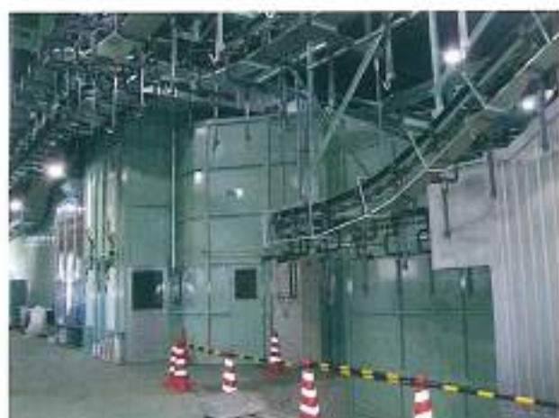
Solvent booth and exit of drying furnace
