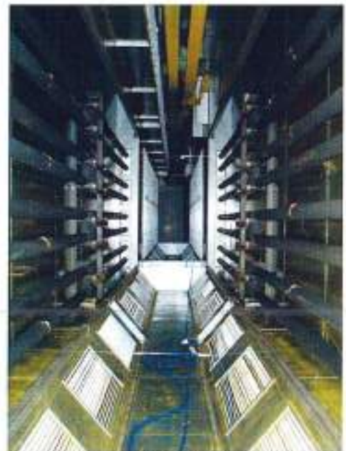
Inside of continuous paint drying furnace for construction machine parts Far-infrared burner BT-33NH x 16 units
