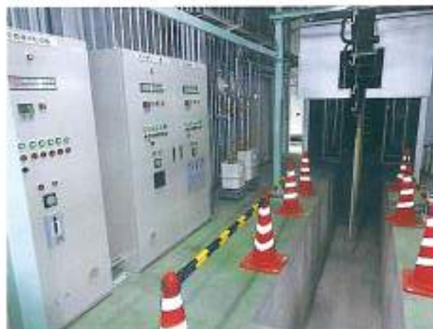
Control panel and entrance of drying furnace
